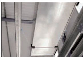
Square Air Ducts
